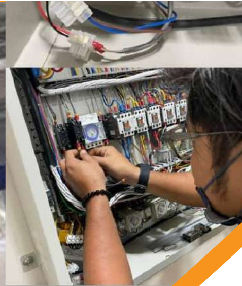
SMARTD CHILLER AIMS D.C
